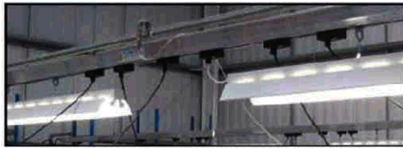
Typical Plugway installation for garment production
