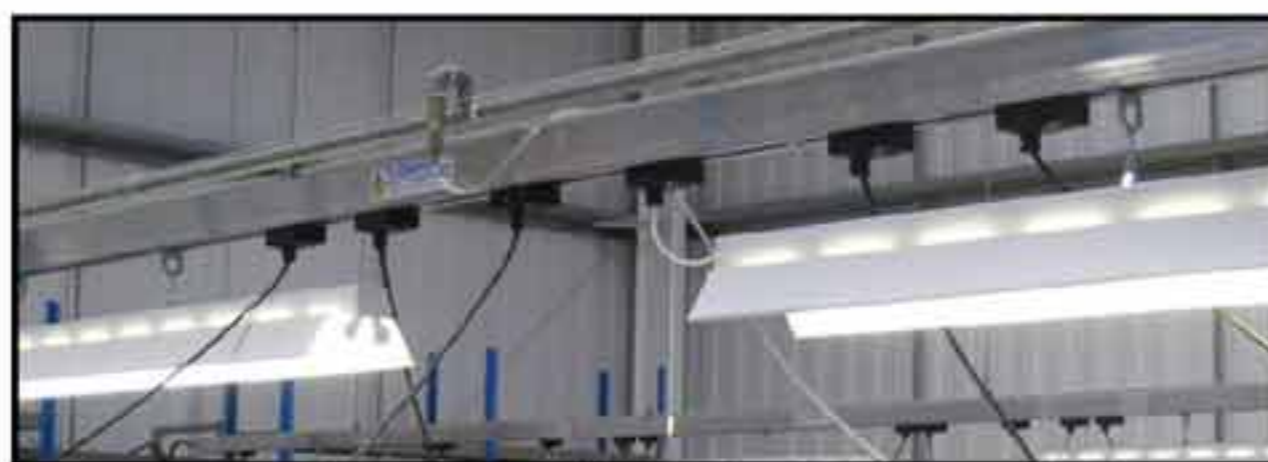
Typical Plugway installation for garment production
